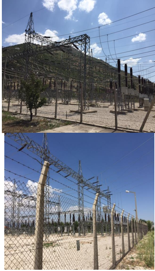
Fig 3. ISPARTA TM high voltage substation measurements
