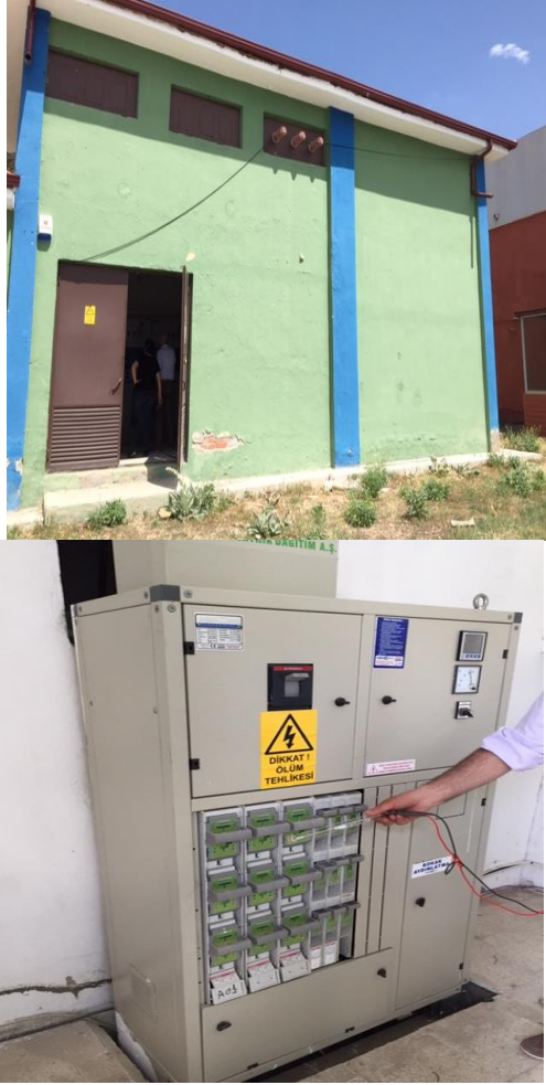
Fig 4. ÇÜNÜR 2 DM distribution center measurements
